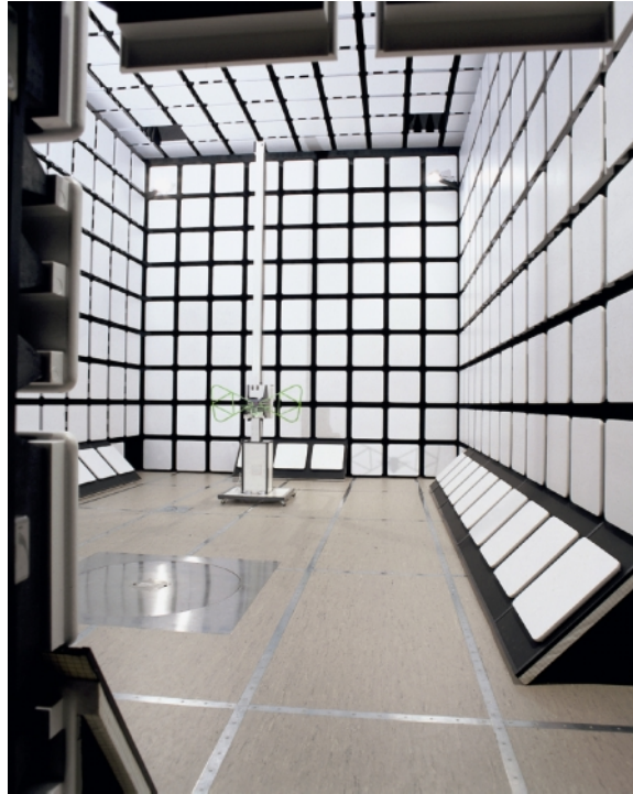
Figure 5: High-Performance Broadband Anechoic Chamber (Photo courtesy of TDK RF Solutions Inc.)
